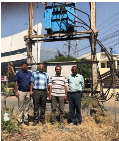
Figure 1. Metering on Proactive Repaired 200 kVA DT
