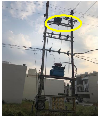
Figure 2. Metering on Proactive Repaired 200 kVA DT
